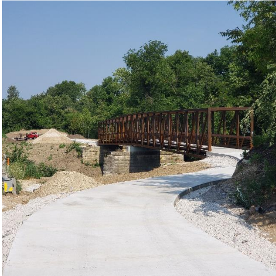
Bridge over Big Creek along the Grant Wood Trail The goal is for the Oxley Rd to Creekside Rd section to be open by the end of August!
