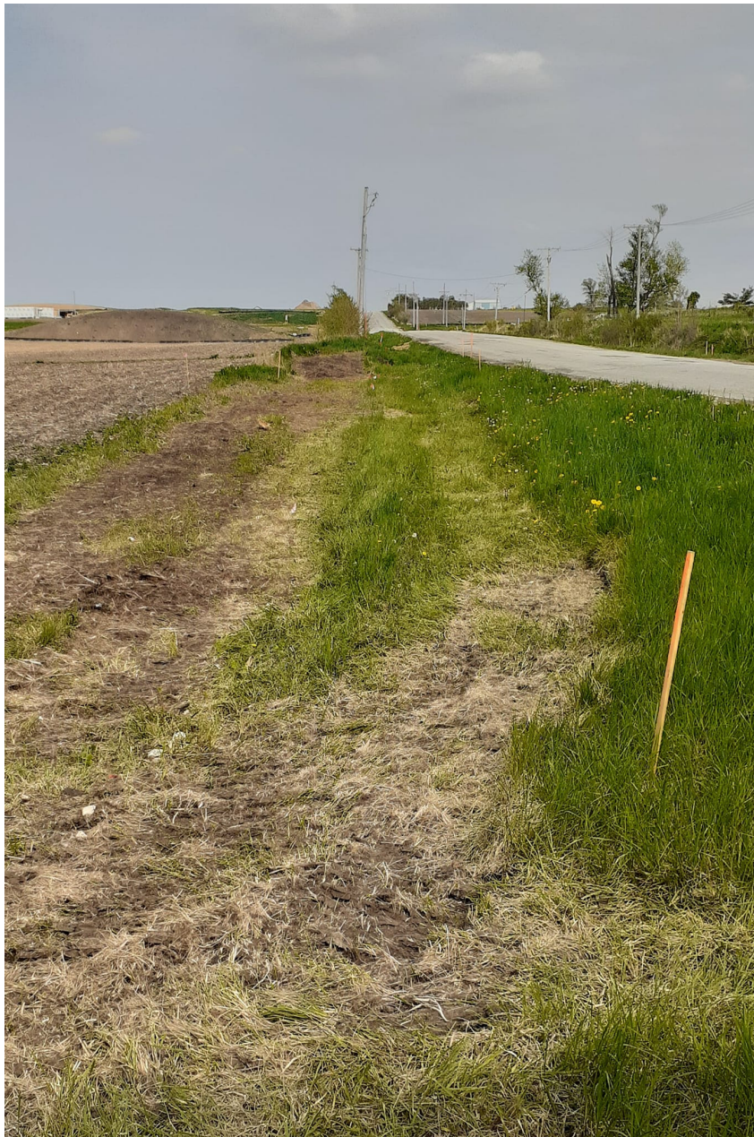
Ground has been broken on Morgan Creek Trail phase III from Morgan Creek Park north to Covington Road. Construction is expected to be completed in 2023 for this segment.
