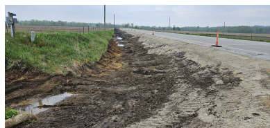
Grant Wood Trail construction alongside Secrist Rd to the new trail bridge and Creekside Rd.
