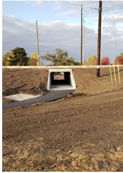
Fresh paving on Grant Wood (aka Lindale) Trail Extension from C Ave to Council Street - Photo below looking north from south side of Blairsferry Underpass! Wow we are under!
